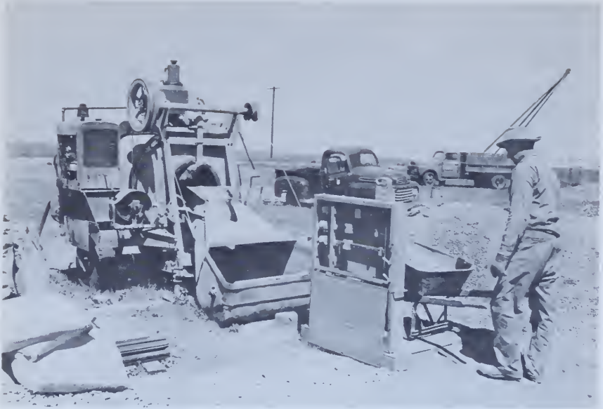
Figure 107.—Batching concrete by means of a portable wheelbarrow scale. Use of such equipment permits securing uniform concrete on the small job. 466-602-604.
